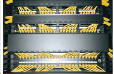
HHCM-1 and HHCM-2 (shown with cabling)
